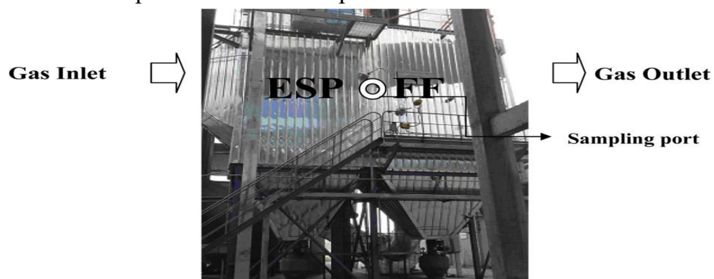
Figure 1. Photograph of the pilot-scale test unit.
