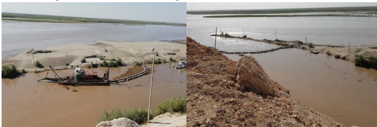
Figure 1. Water intake structure from the Amudarya River to the Karshi Main Canal
